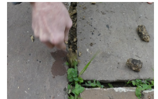
Remove organic material and loose jointing. Jet wash clean.
